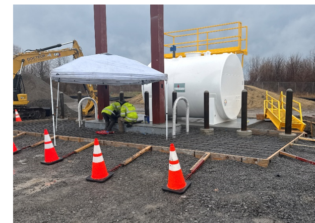
Fuel Island at New Transportation Facility
